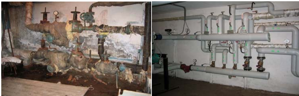
Heat substation before upgrade (left) and after (photo courtesy of ENSI)
